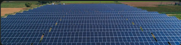
2.5 MW DC / 2 MW AC Solar Plant LOHARU, HARYANA
