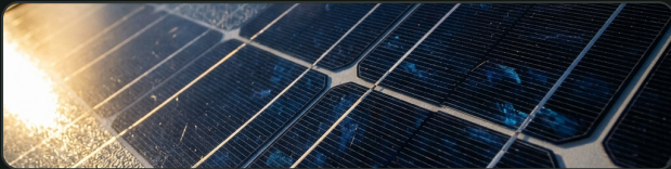
2.5 MW DC / 2 MW AC Solar Plant PAHARI MANDIR, HARYANA
