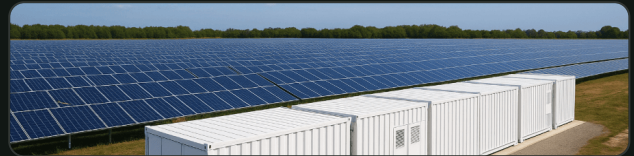
2.5 MW DC / 2 MW AC Solar Plant DIGAWAN, HARYANA
